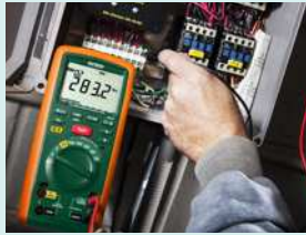
Voltage check on motor starter
