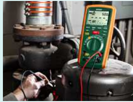
Insulation test on pump motor
