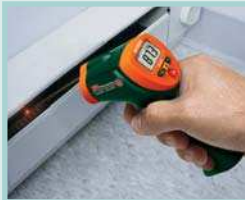
Test for temperature in heating systems
