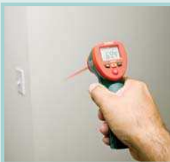
Check building for insufficient insulation
