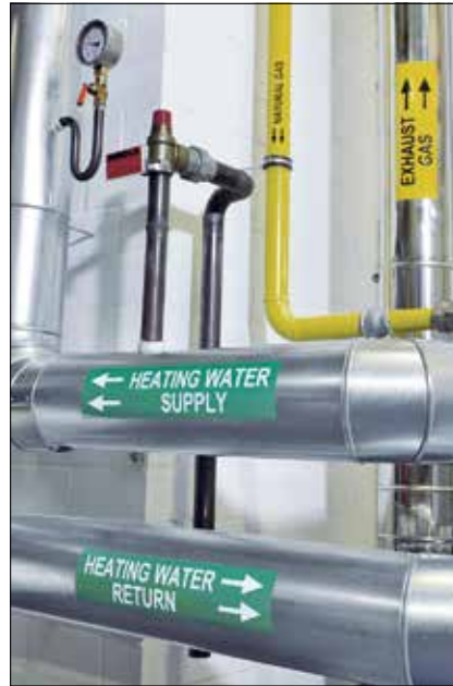
Large and highly visible pipe marking.
