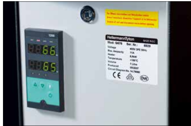
Professional type plate on a heating unit.
