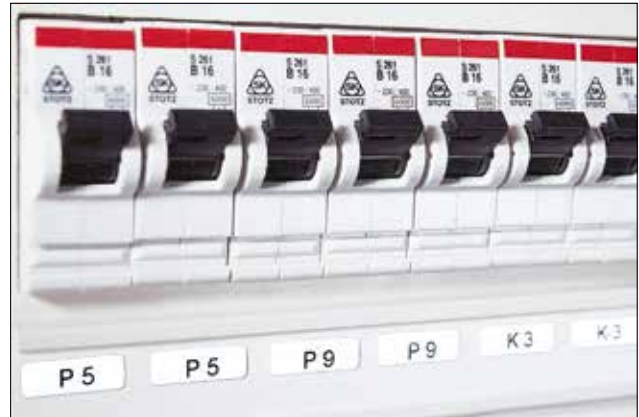
Clear and permanent identification of switch gears.
