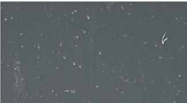
The joint has only been altered at isolated points by the UV-radiation.
