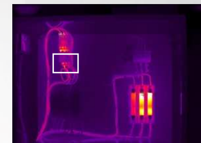
Full image, taken from 5 feet away with a TiX1000 infrared camera. The area shown in the white box is blown up below.
