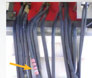
Power Distribution-Full visible
