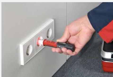
Test wall sockets for AC voltage and polarity
