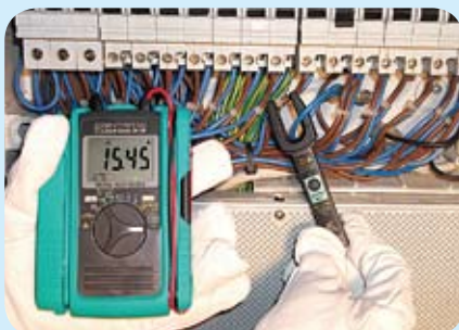
Measuring current in a Switchboard
